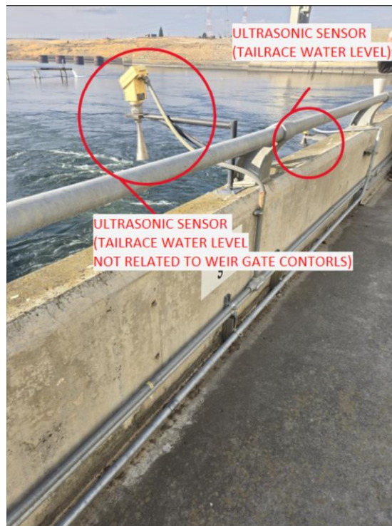
Figure 10: SFE1 & 2 Tailrace Water Level Sensors
