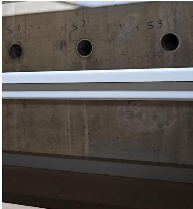
Figure 5: Undocumented Embedded Conduits Bay 1 Middle Tray
