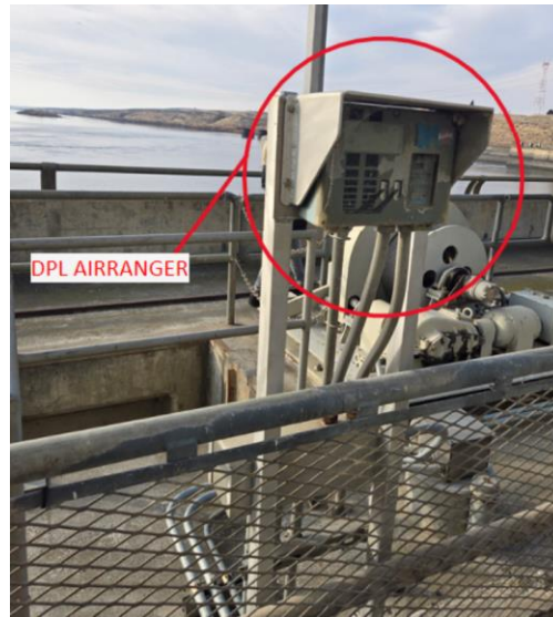
Figure 16: Central Weir Gate Sensor & Devices
