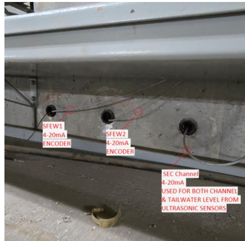
Figure 13: Fishway Gallery Embedded Control Conduits
