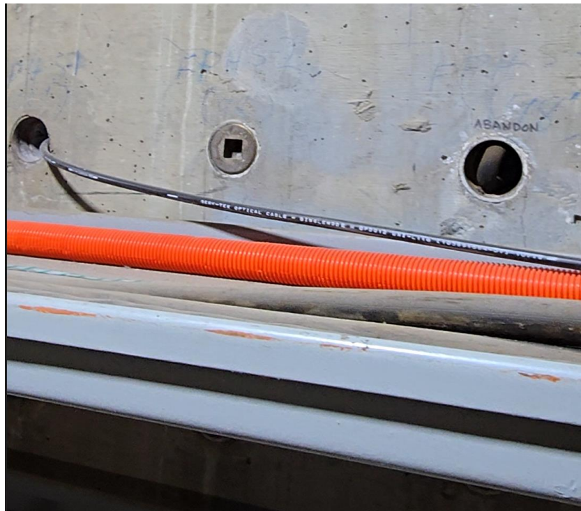
Figure 4: Undocumented Embedded Conduits Bay 1 Top Tray
