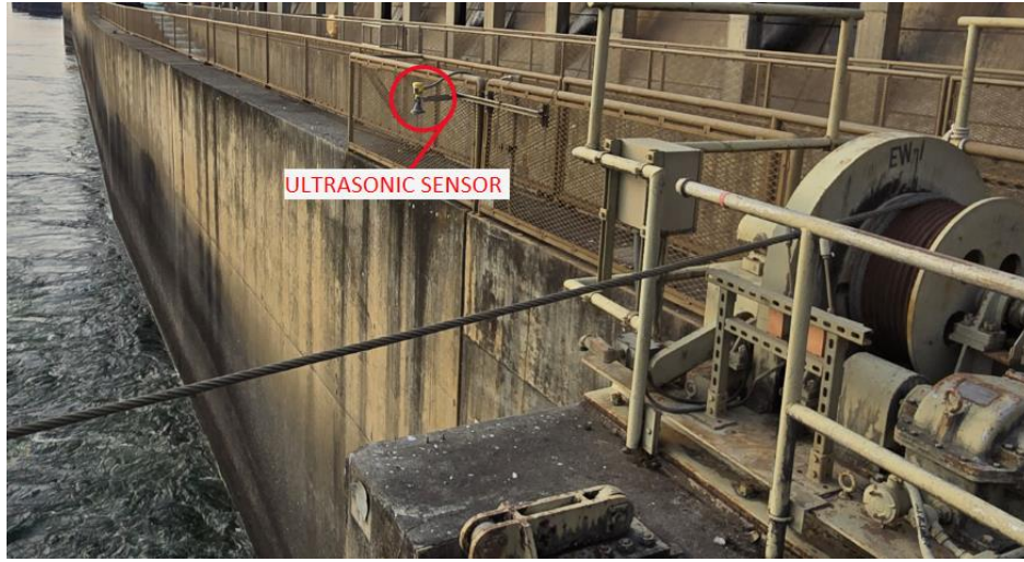
Figure 22: North Fishway Tailrace Ultrasonic Sensor
