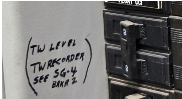
Figure 2: CRA4 Panel In FCQ4, Breaker 13
