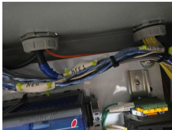
Figure 20: Central PLC Control Cables
