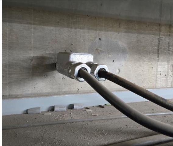
Figure 1: FCQ1-r1-CC1 Junction Box
