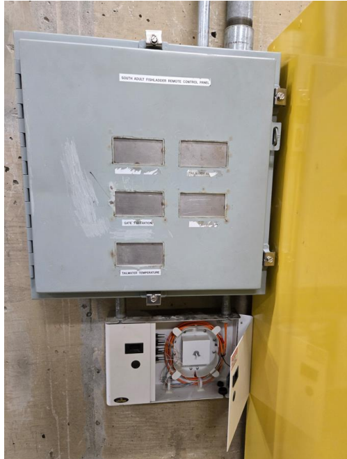
Figure 15: SFE PLC Enclosure
