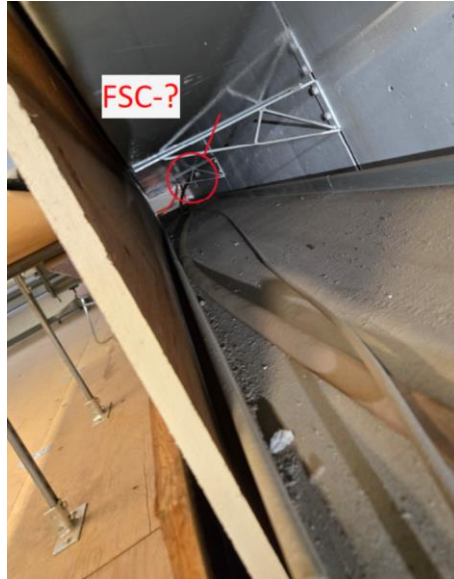
Figure 6: Undocumented FSC Embedded Conduit
