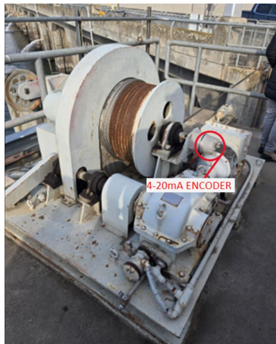
Figure 12: SFE1 Hoist Equipment (Typical for all locations)
