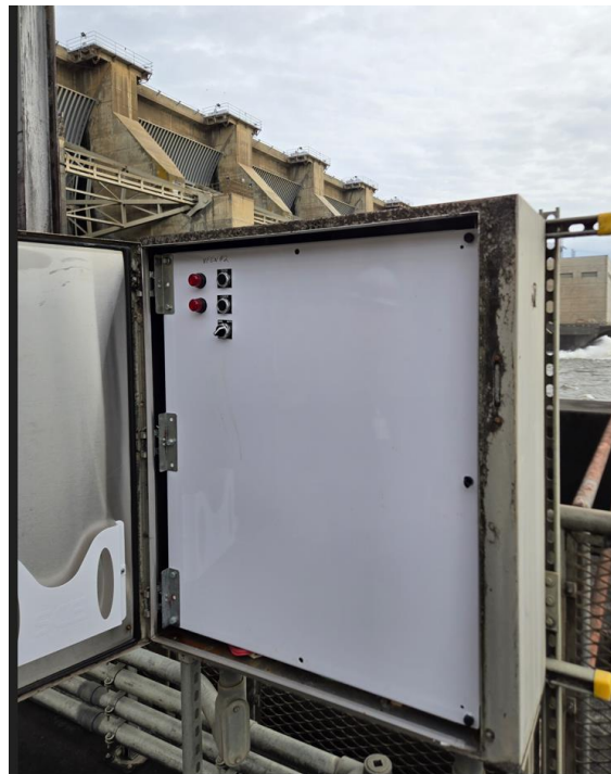
Figure 27: NFEW2 Control Enclosure
