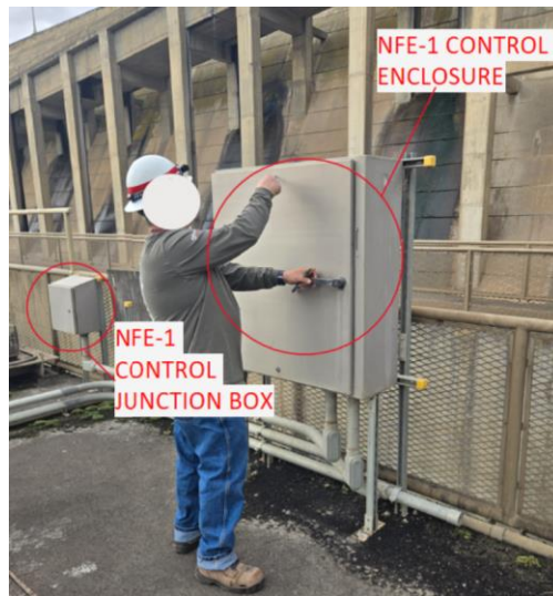
Figure 28: NFE1 Control Enclosure
