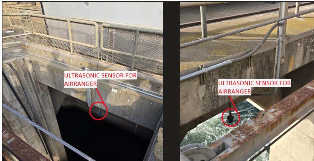
Figure 17: Central Weir Gate Ultrasonic Sensors
