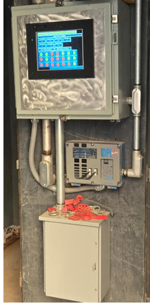
Figure 26: North Fishway HMI/PLC Cabinet In FCQ4 Shack
